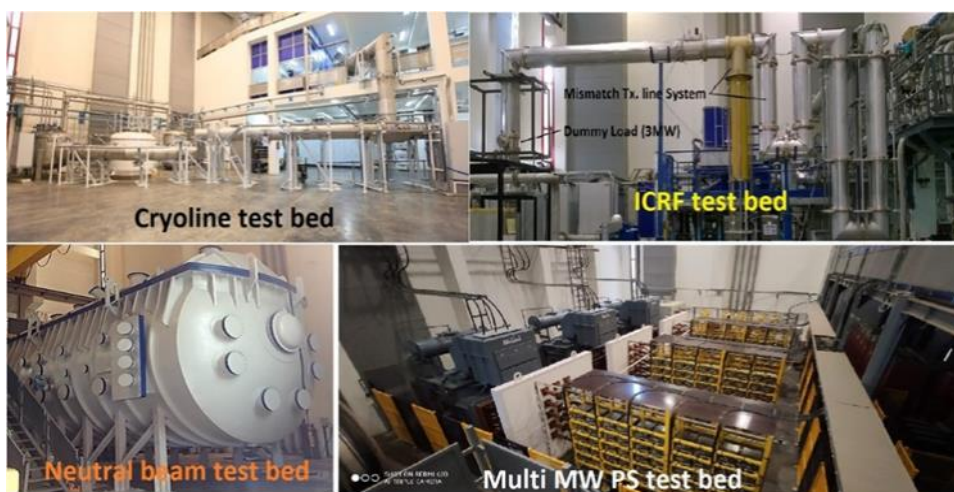
Figure 3: The various test beds in ITER India laboratory for development of Cryolines, RF sources, Neutral beam and Multi MW power supplies
