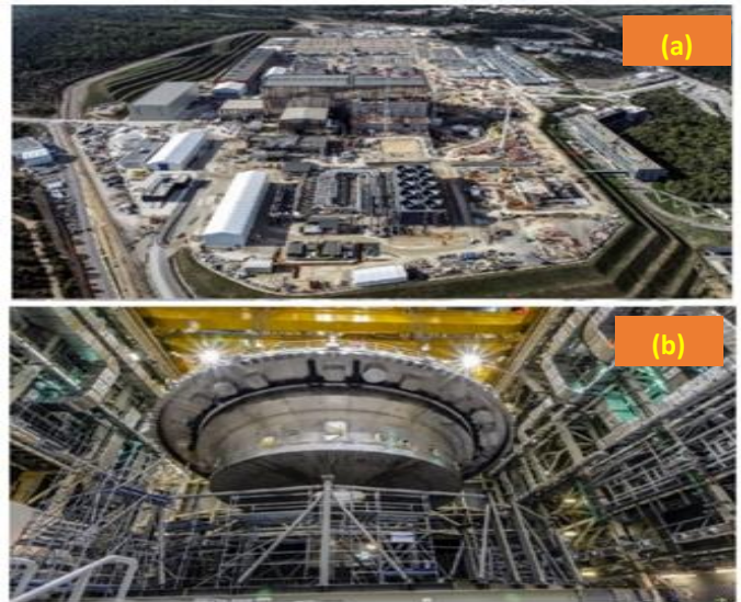
Figure 2: a) ITER site with 75% activities completed, b) Base section of the cryostat supplied by India being moved for installation in ITER Tokamak pit, first and the heaviest component to be installed
